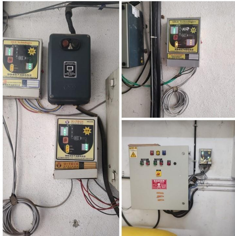
Figure 4-4: Water level controller for Basement to overhead tank water pumping
