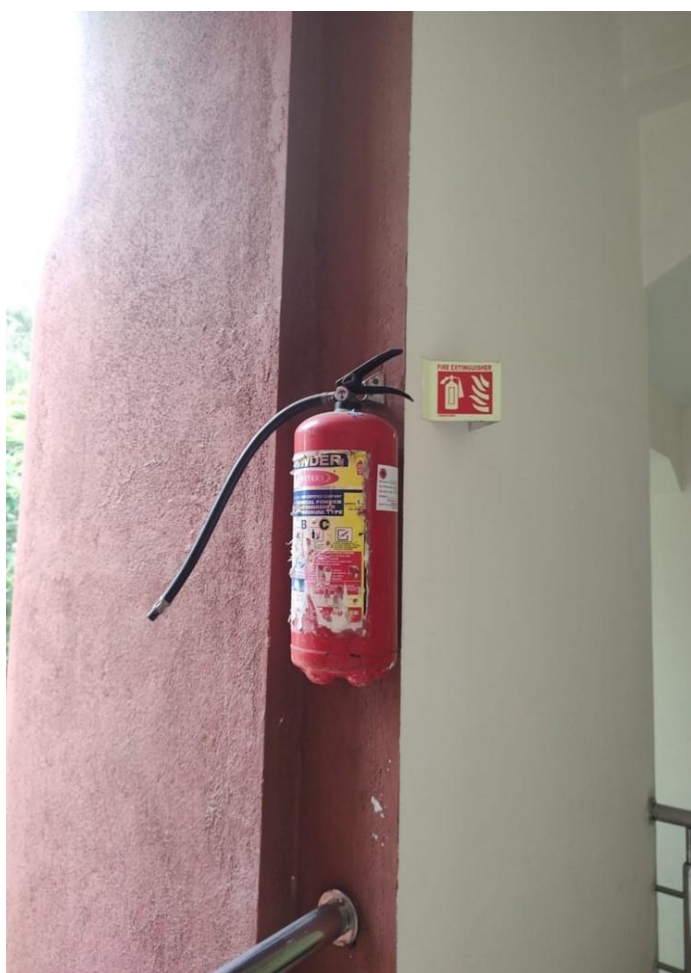
Figure 3-1: Fire Extinguisher installed in the floors
