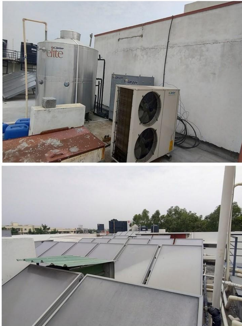
Figure 4-6: Heat pump and solar water heater installed in the college
