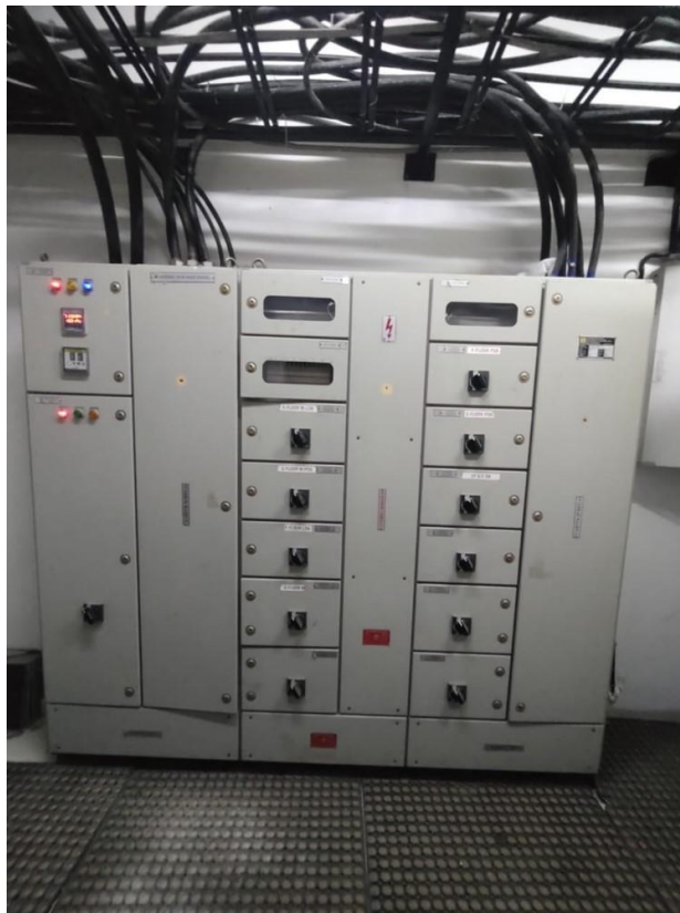
Figure 5-2: Electrical Panel room
