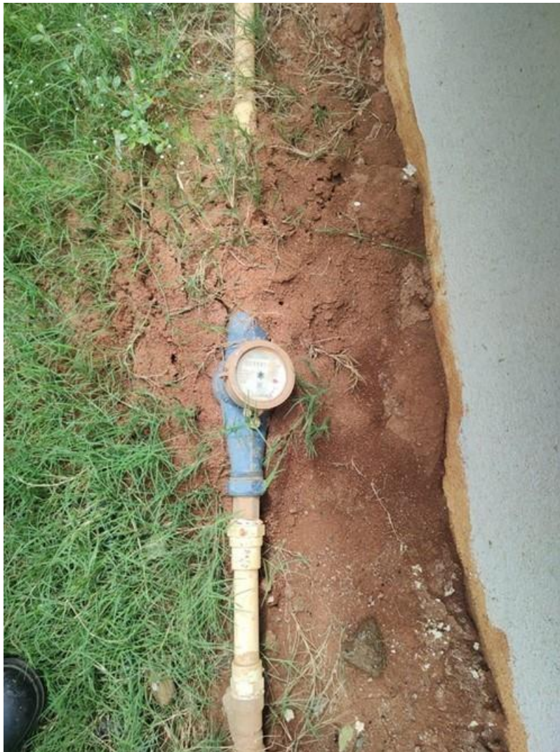
Figure 4-7: Water flow meter
