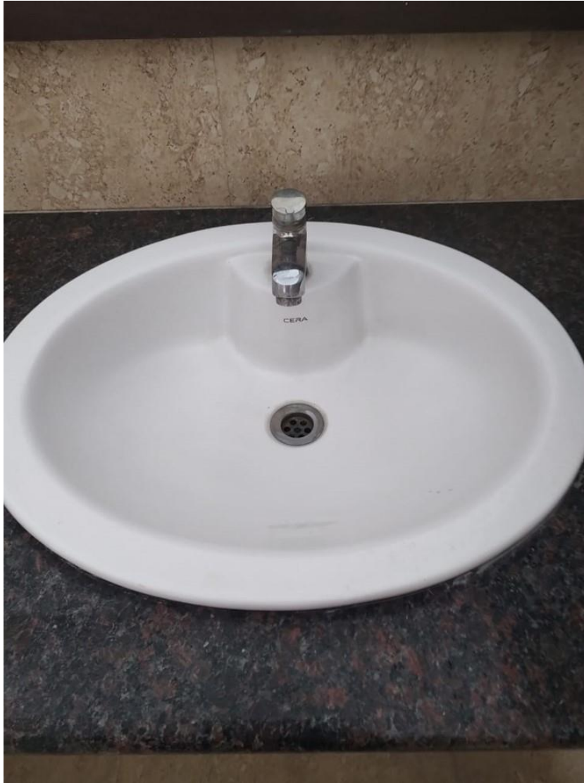
Figure 4-10: Sample photo of push type tap in the wash rooms
