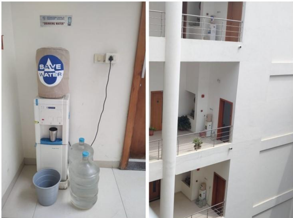
Figure 4-5: Drinking water dispenser available in floors
