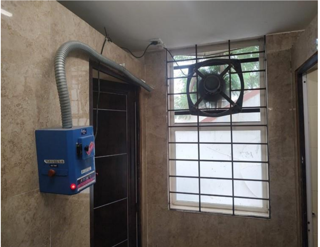
Figure 6-4: Sanitary napkin incinerator installed in girls rest room
