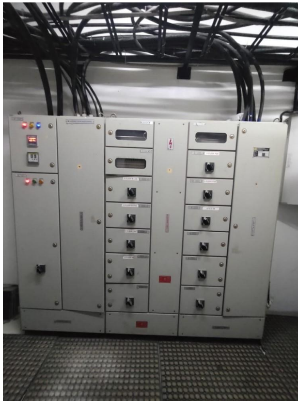
Figure 5-2: Electrical Panel room
