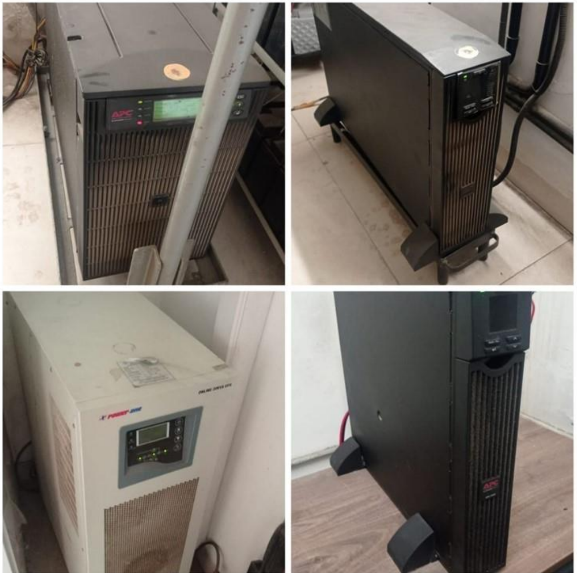
Figure 5-10: UPS and batteries
