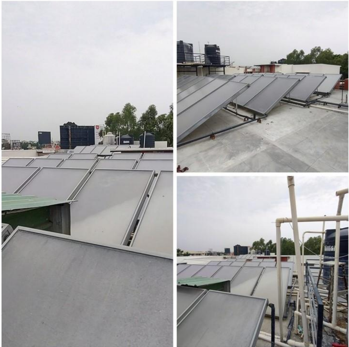
Figure 5-9: Use of Solar Water Heater
