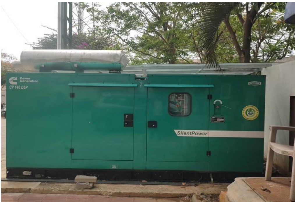
Figure 5-3: Diesel Generator (DG) sets
