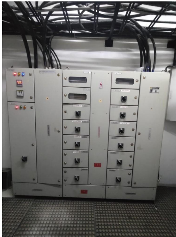
Figure 5-2: Electrical Panel room
