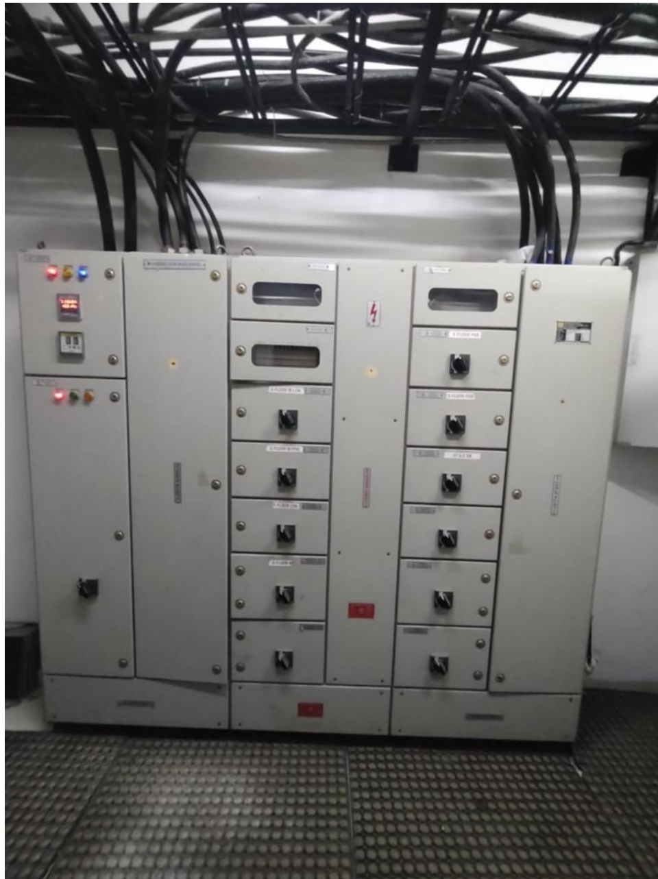
Figure 5-12: Electrical safety mats near electrical panel
